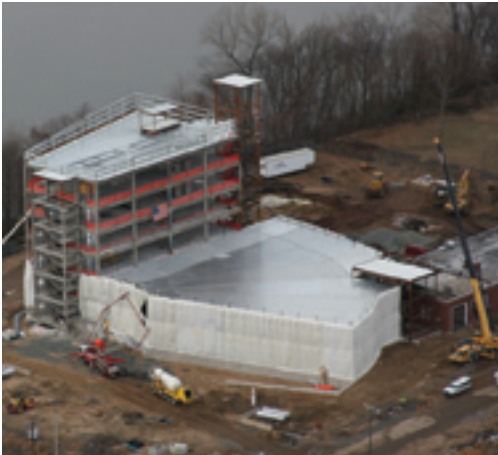
Goodwin College constructed their new River Campus along the Connecticut River in East Hartford with financing from NewAlliance Bank.
